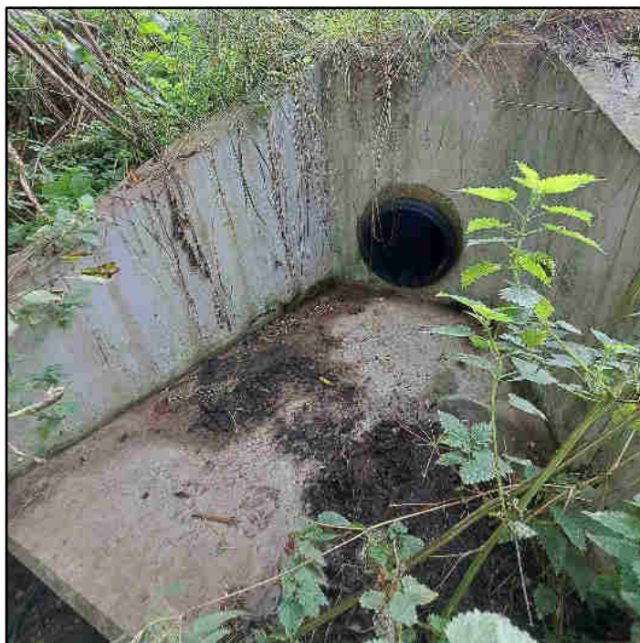
Photograph 11: Pond Overflow Outflow Pipe, showing Lack of Guard
