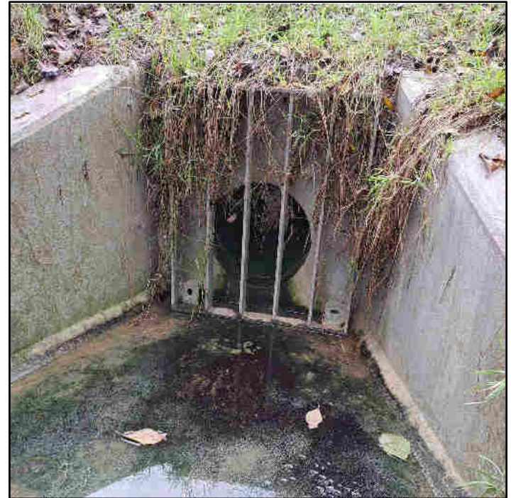
Photograph 10: Drainage Inflow Pipe from Artificial Sports Field
