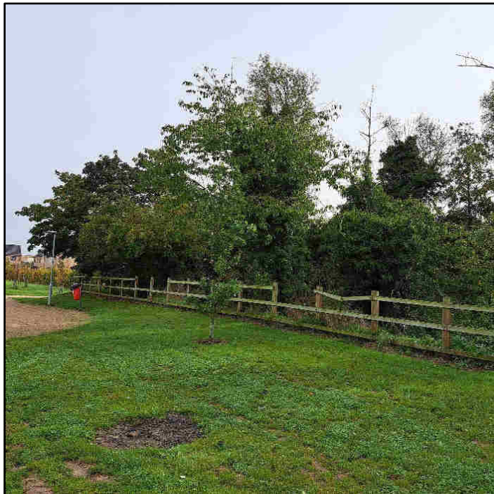
Photograph 3: Fence Around Kingfisher Pond, Showing Broken Sections
