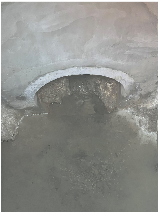
Figure 1: Water ingress from S418ST in Chamber S419
